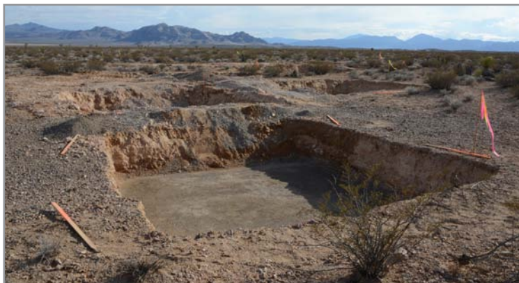
Seven Magic Depressions: The foundations for the rock stacks being prepared before installation. CLUI photo
