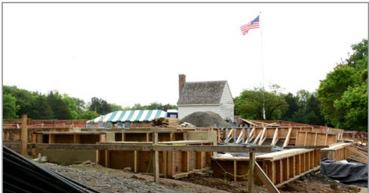
George Washington's childhood home at Ferry Farm, being built from scratch in 2016-2017, will float above the ground on a special cantilevered foundation so as not to disturb the archeological integrity of the original home site beneath it. CLUI photo
