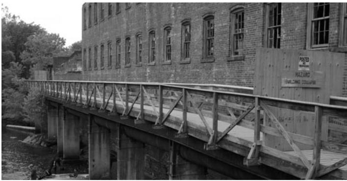
Part of the collapsing Tioronda Hat Works mill complex, on Fishkill Creek. CLUI photo
