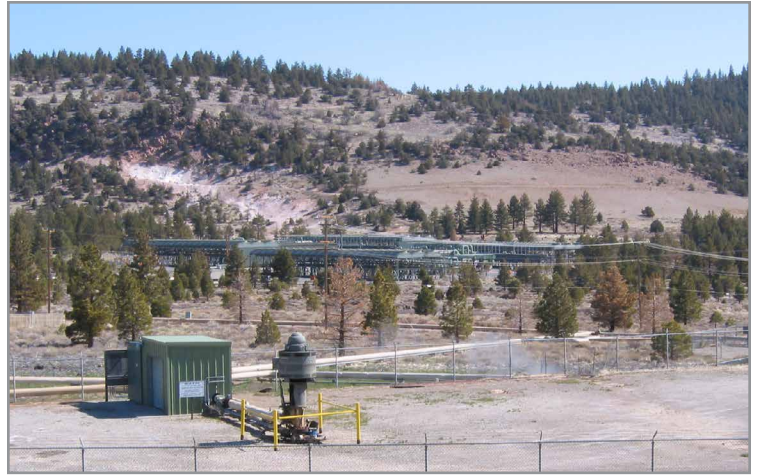
Geothermal plants at Mammoth.
