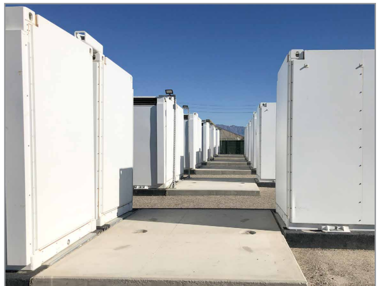
Rows of boxes of batteries in Satcoy, near Ventura, California, at a battery storage project with a 100-megawatt output capacity. CLUI photo
