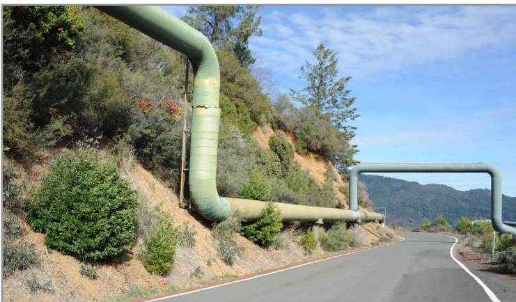
Distribution pipes at the Geysers.
