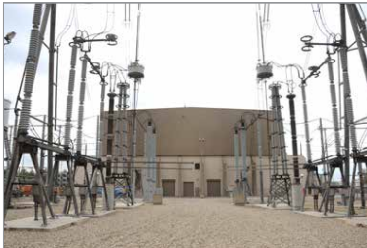
The DC line from the Pacific Intertie enters symmetrical Valve Halls at the Sylmar Converter Station. CLUI photo
