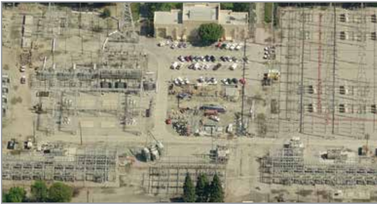
Receiving Station B, on Central Avenue, is one of 23 DWP receiving stations, where power enters the grid from its various sources. Voltage is usually stepped down at the receiving stations, and is distributed to clusters of smaller substations, known as distributing stations. Bing photo
