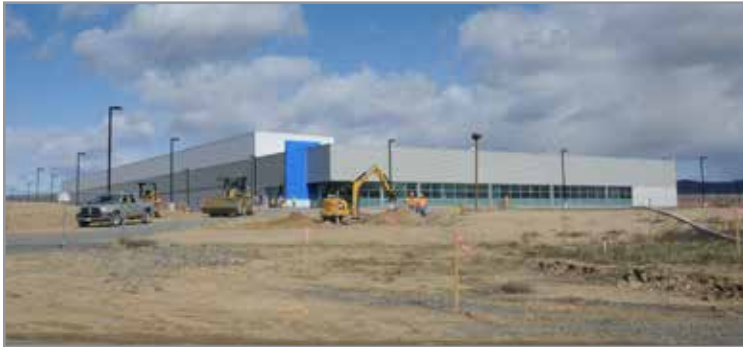
Vantage, a data center company, built its first data center outside Santa Clara in Quincy, Washington, in 2012, joining Dell, Microsoft, Sabey, and Yahoo in this remote eastern Washington town. CLUI photo
