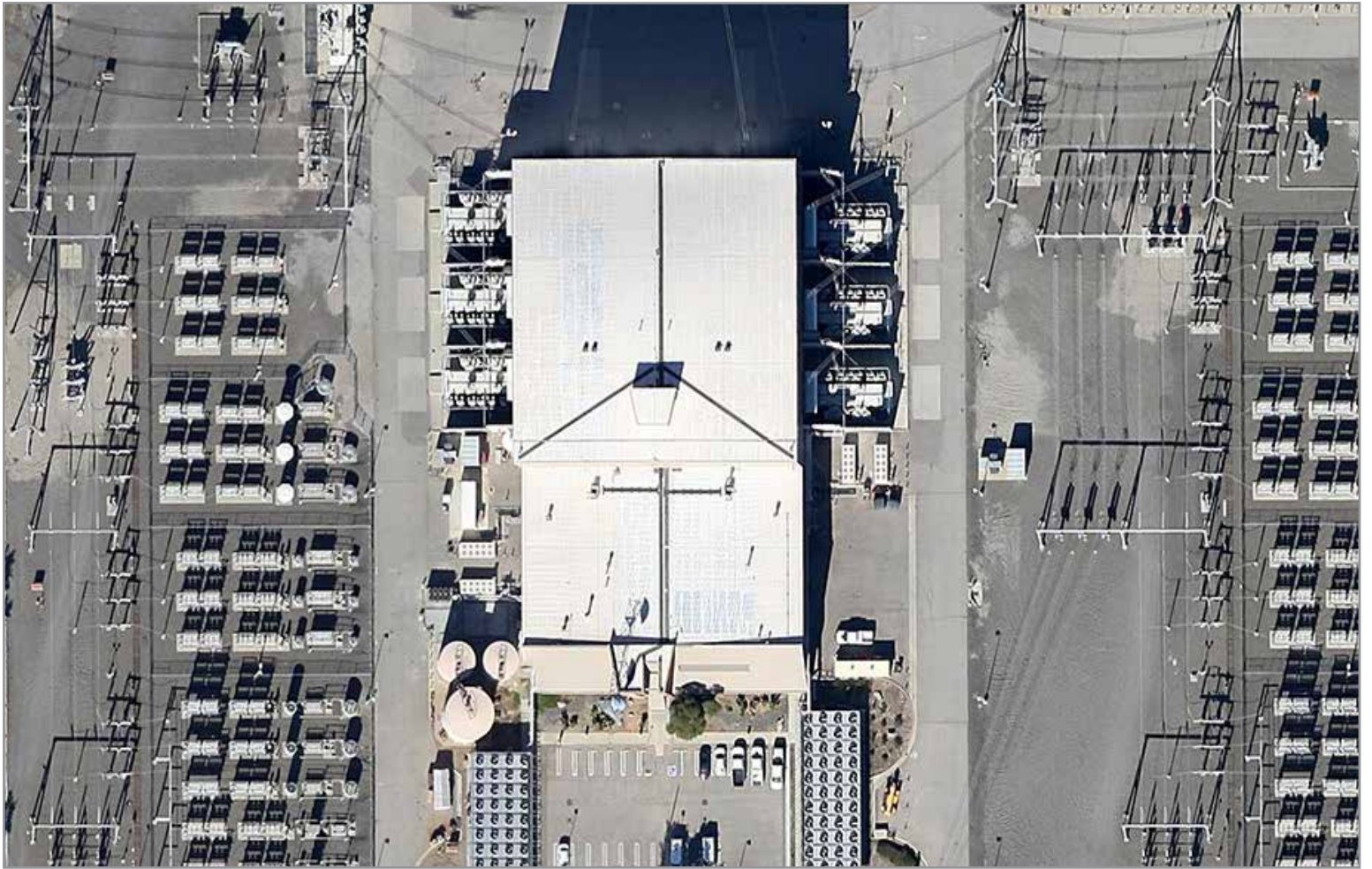
The East Sylmar HVDC Converter Station.
